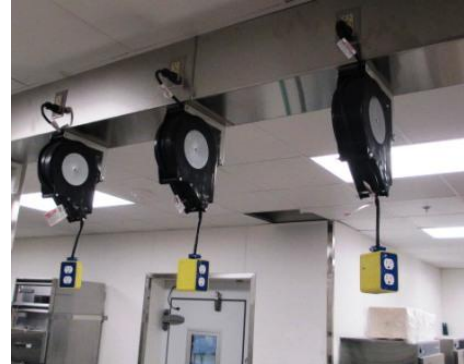
Power Cable Reel
