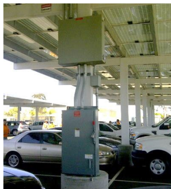
Column Mounted Equipment
